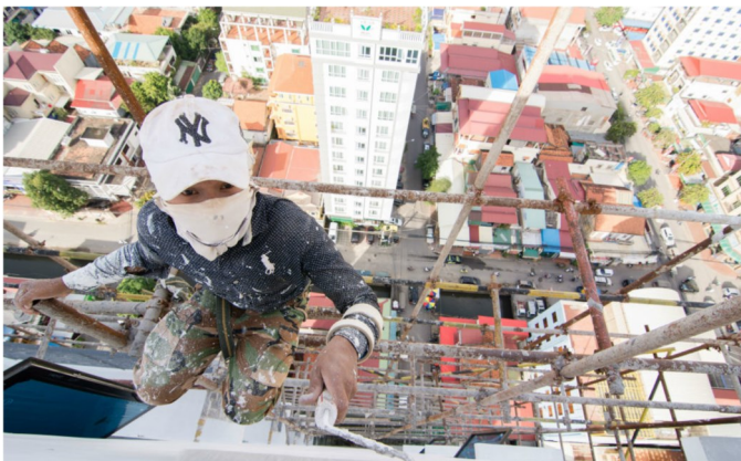
A painter painting a highrise building in Phnom Penh without any security gear. Photo Alex Consiglio
