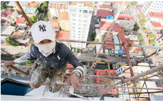
A painter painting a highrise building in Phnom Penh without any security gear. Photo Alex Consiglio
